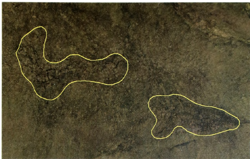
Figure 1: Frost cracking and re-wire ice formation.
